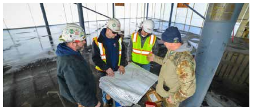
Construction workers review blueprints for the Capital Area Multimodal Gateway, operated by CATA.
