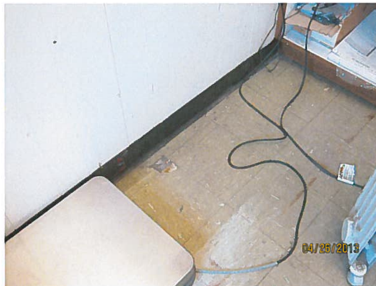
Photograph No. 2 HA-8 Amtrak Building Greyhound Office 9"X9" Gray Floor Tile 3% Chrysotile asbestos
