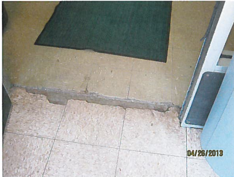
Photograph No. 1 HA-2 Amtrak Building Waiting Area 9"X9" Green Floor Tile 3% Chrysotile asbestos
