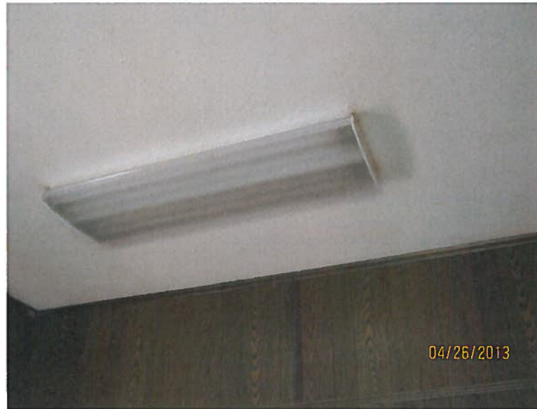
Photograph No. 9 Fluorescent Light Amtrak Station
