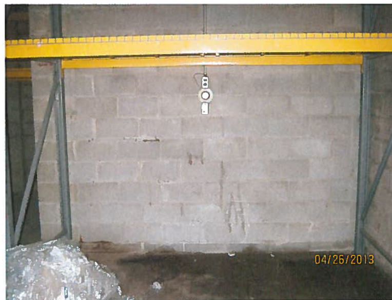
Photograph No. 6 Mercury Thermostat Storage Building A 3 rd East Bay and Floor Staining
