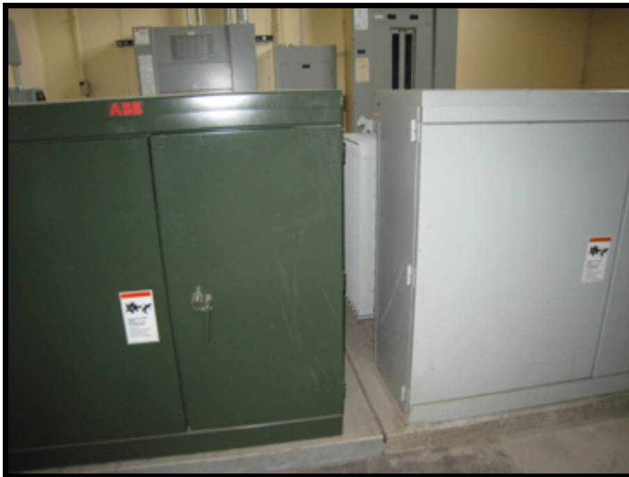
Photograph No. 10 View of Building 2 – interior – utility room - pad-mounted transformers
