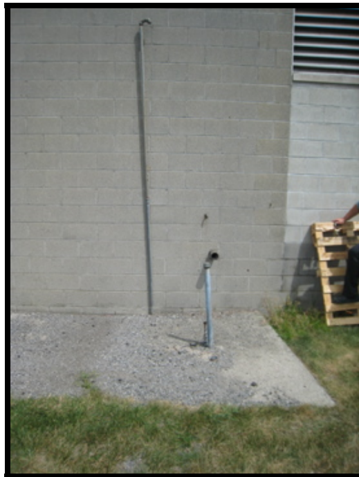
Photograph No. 20 View of subject property exterior – fill port/vent pipe (550-gallon heating oil UST)
