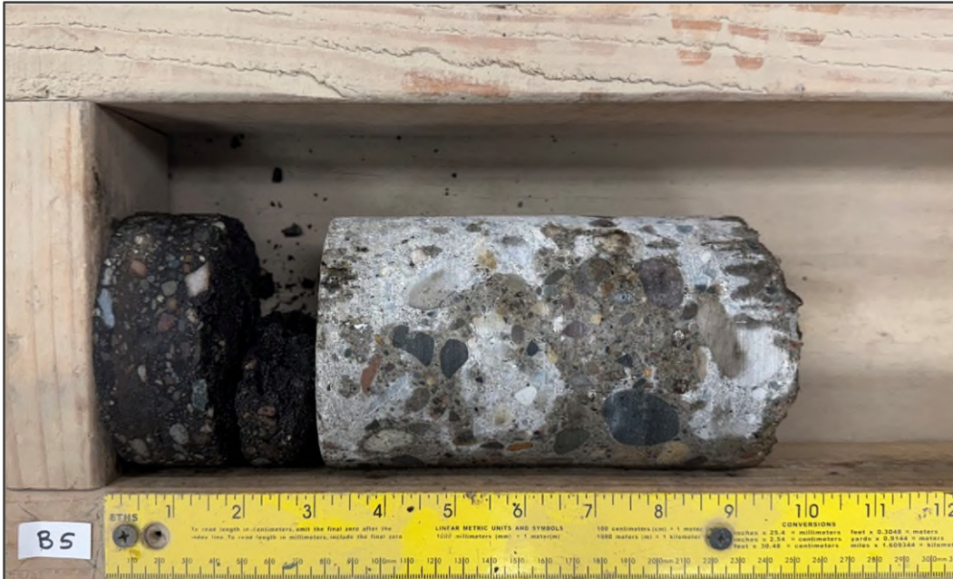
PHOTO NO. 5: Boring P5 - 3 inches of Asphalt and 7 inches of Concrete
